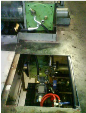
Installation kylaggregat Pressgrannar Nrkp
